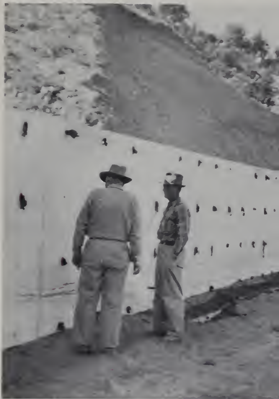
Figure 178.—Repairing cone-bolt holes in a bench-f packed with wet burlap in the afternoon and the mortar the next morning. This is a second filling of cause improper procedure caused unsatisfact filling. PX-D-33056
